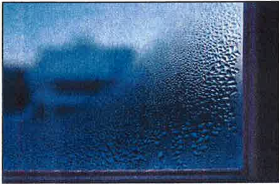
Condensation on the inside of a windowpane.
